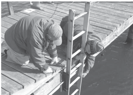
Howard Millard & Ken Kaim install a safety ladder at the April 4th work party.
